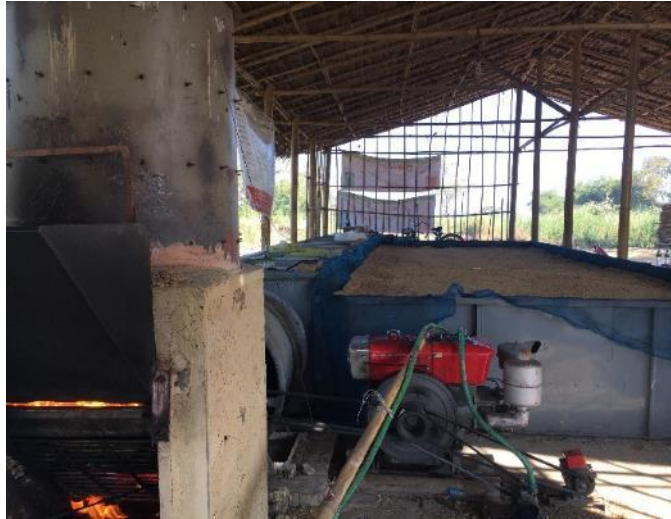
Flat-bed dryer powered by rice husk furnace
